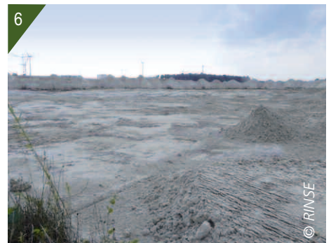
3. 4. The colonised pond, prior to the work. 5. Dredging work. 6. Site following the work.
